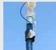
Shut Off valve in pipeline
