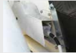
LIMIT SWITCH HOPPER GRID
